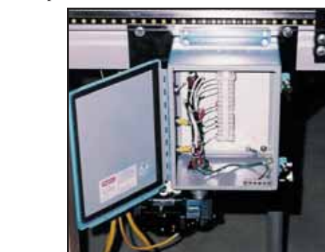
Electronics: Typical pre-wiring of components to local junction boxes
